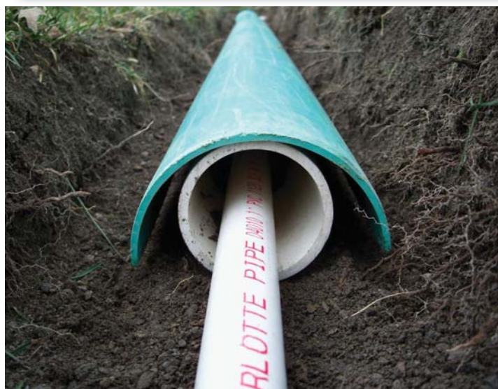
Low pressure distribution system in the expanded shale leach bed.
